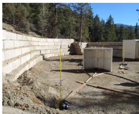
A view of the Project 2 setup.
